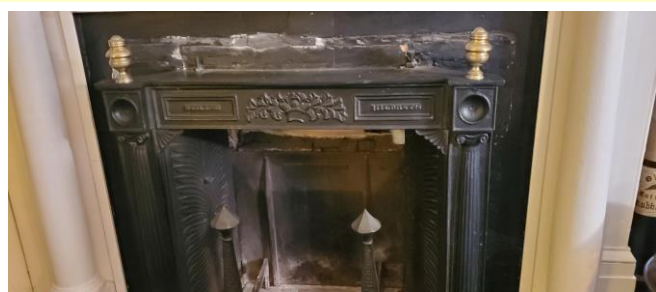
Photo shows the brass finials atop the pillars on the exterior of the fireplace insert
