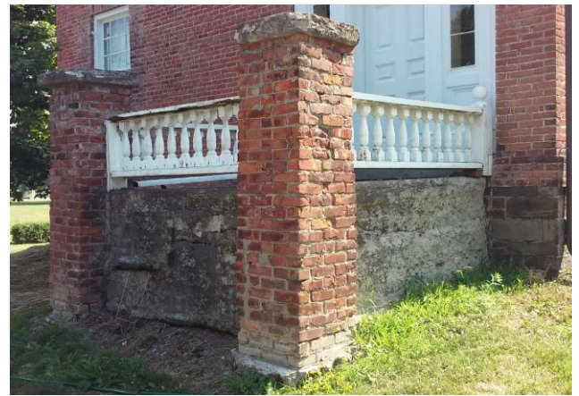
West deck in 2018 showing broken brick, rotted balustrade
