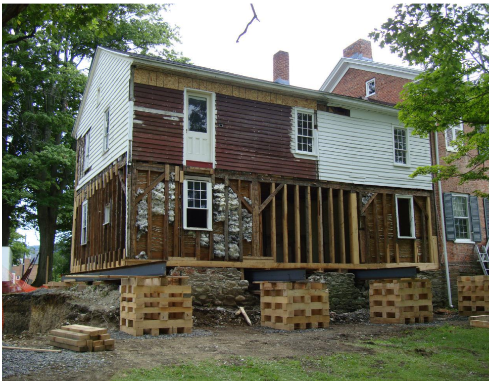
East Addition resting on steel beams in preparation for excavation of a new basement. Note the new sill plates, posts and studs. Summer 2013
